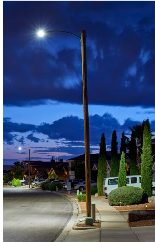
Cobra head light mounted on wooden pole.
